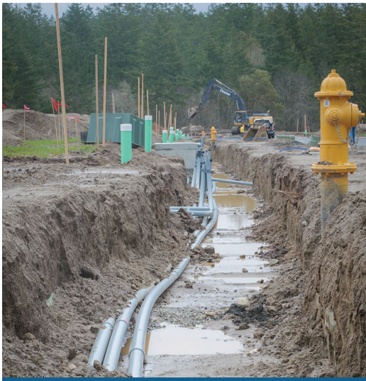
The joint-use trench for the Madrona Ridge subdivision includes conduit for electric and telecom services.
