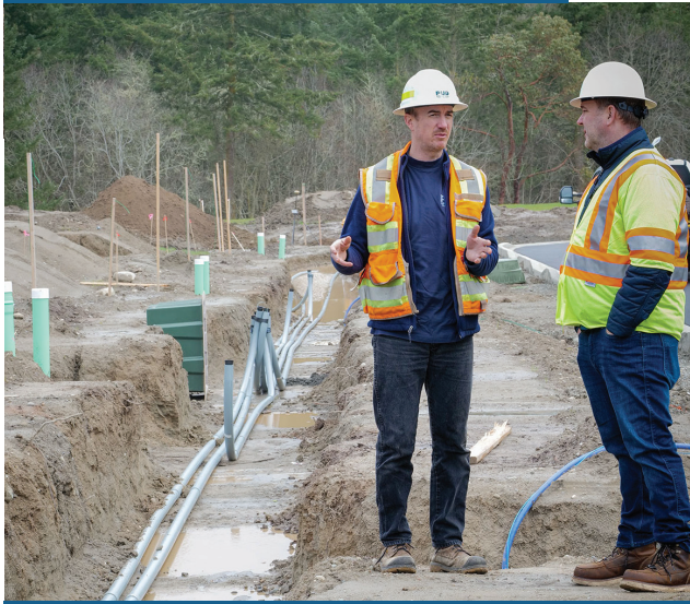
Staking Engineer, Russell Miller (left) discussing joint-use trench layout with PUD Safety Manager, Jeff Dodd.
