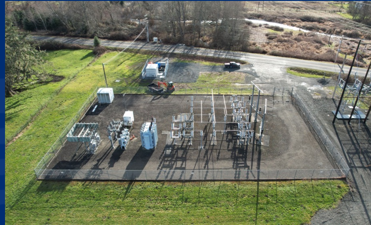
SHOWN: Quilcene Substation
